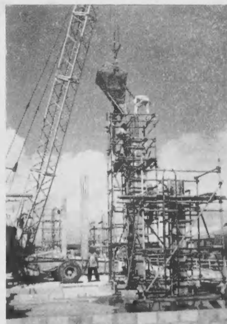
Another cubic yard of concrete goes into the columns being poured at the new Retail Commissary west of the Main Gate. Good progress is being made on the job, with all columns finished in the Cold Storage area and part in the Retail area. Next step will be the extensive carpentry work of building the wood forms into which cement will be poured to make the roof.
